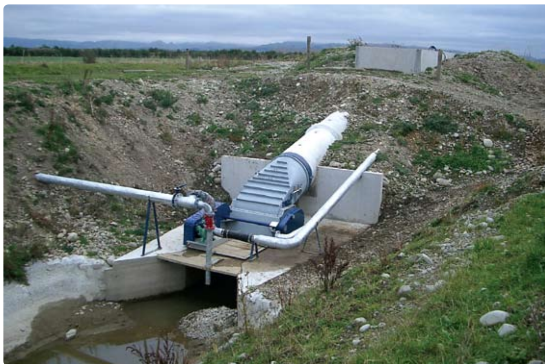
Hydro-powered irrigation in operation in Canterbury. Photo courtesy Crosstech Engineering.
