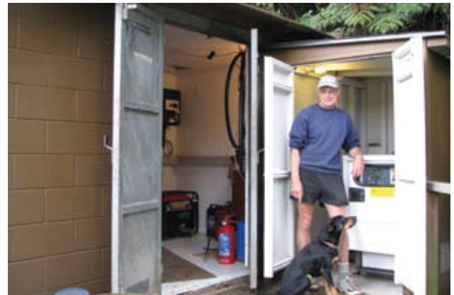
The diesel generator shed.
