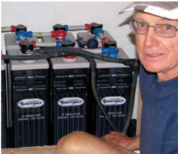
The battery bank.
