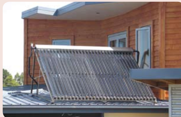
The solar collector raised to be more square-on with the low winter sun
