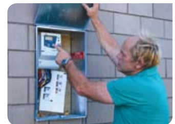
The two-way electricity meter, which measures how much is imported and exported.
