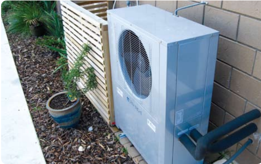
Heat pump water heaters provide hot water for the lodge.
