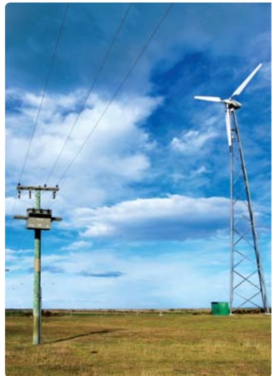
The turbine at Southbridge, Canterbury generates 200,000kWh per year.
